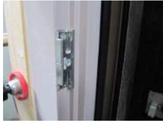
Photo 32 Locking situation, frame member / sash member
