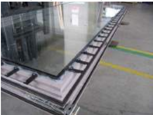
Photo 23 View of horizontal glazing rebate, additional sealed with pourable sealant
