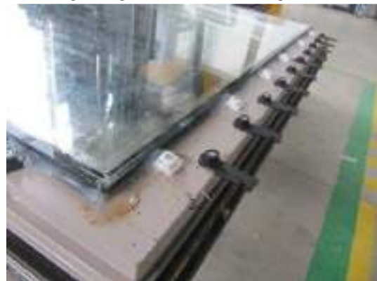
Photo 24 View of horizontal glazing rebate, additional sealed with pourable sealant
