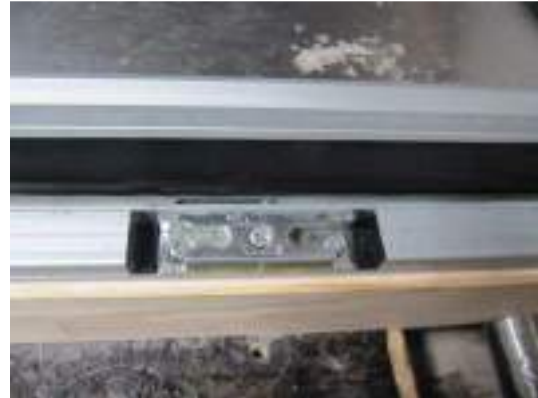
Photo 34 Locking situation, frame member / sash member
