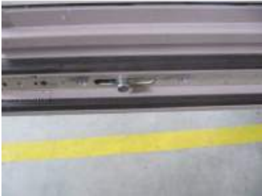
Photo 33 Locking situation, frame member / sash member
