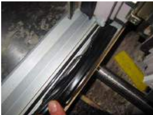
Photo 11 Threshold seal, additional sealed with pourable sealant horizontal at bottom and lateral
