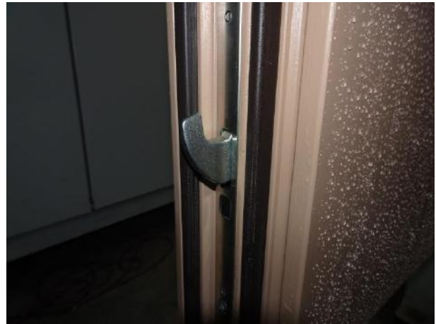
Picture 20 Auxiliary lock
